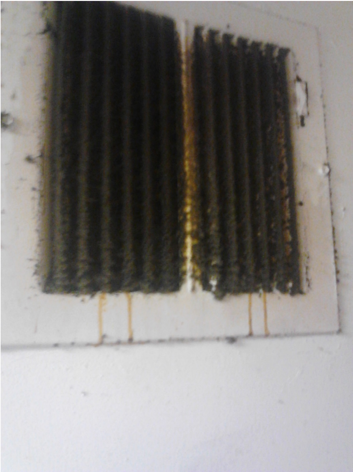
Vent in client's kitchen (same apartment as shown in Exhibit B-3 and Exhibit B-4).
