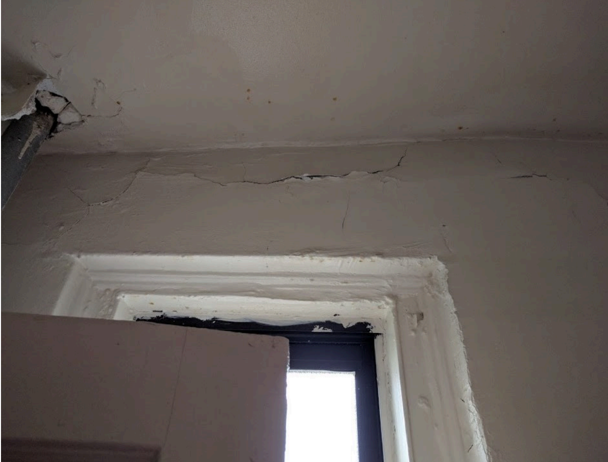
Significantly damaged ceiling and walls in client's bathroom.
