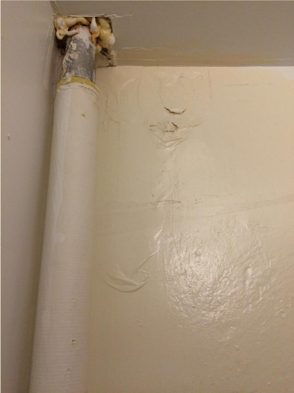
Damaged ceiling and walls.
