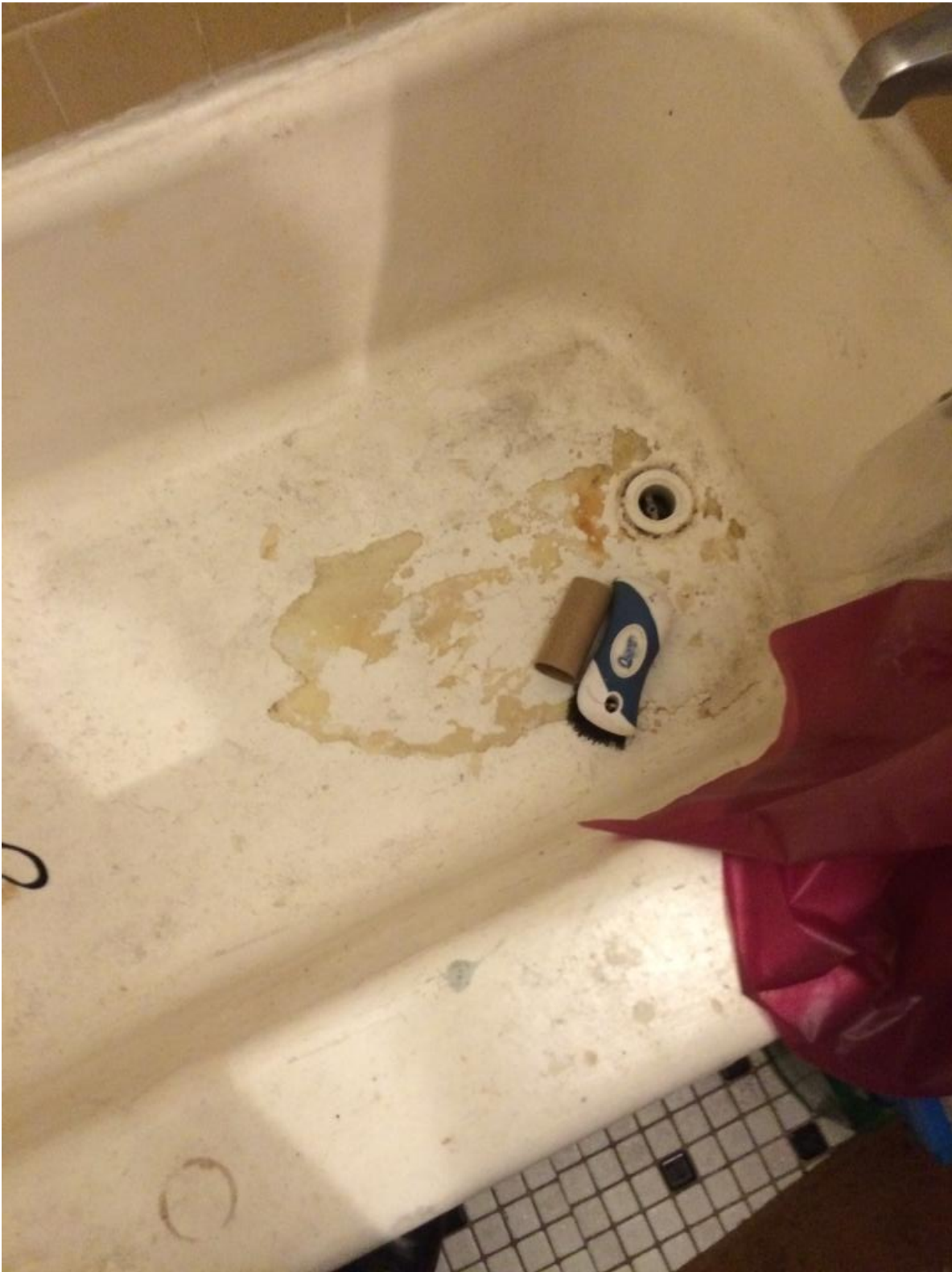
Client's bathtub (same apartment as shown in Exhibit B-6 and Exhibit B-7).
