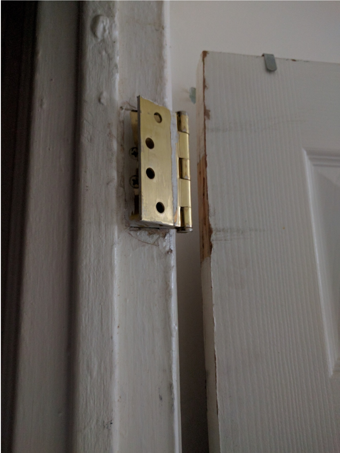
Client's bathroom door detached from its hinges.
