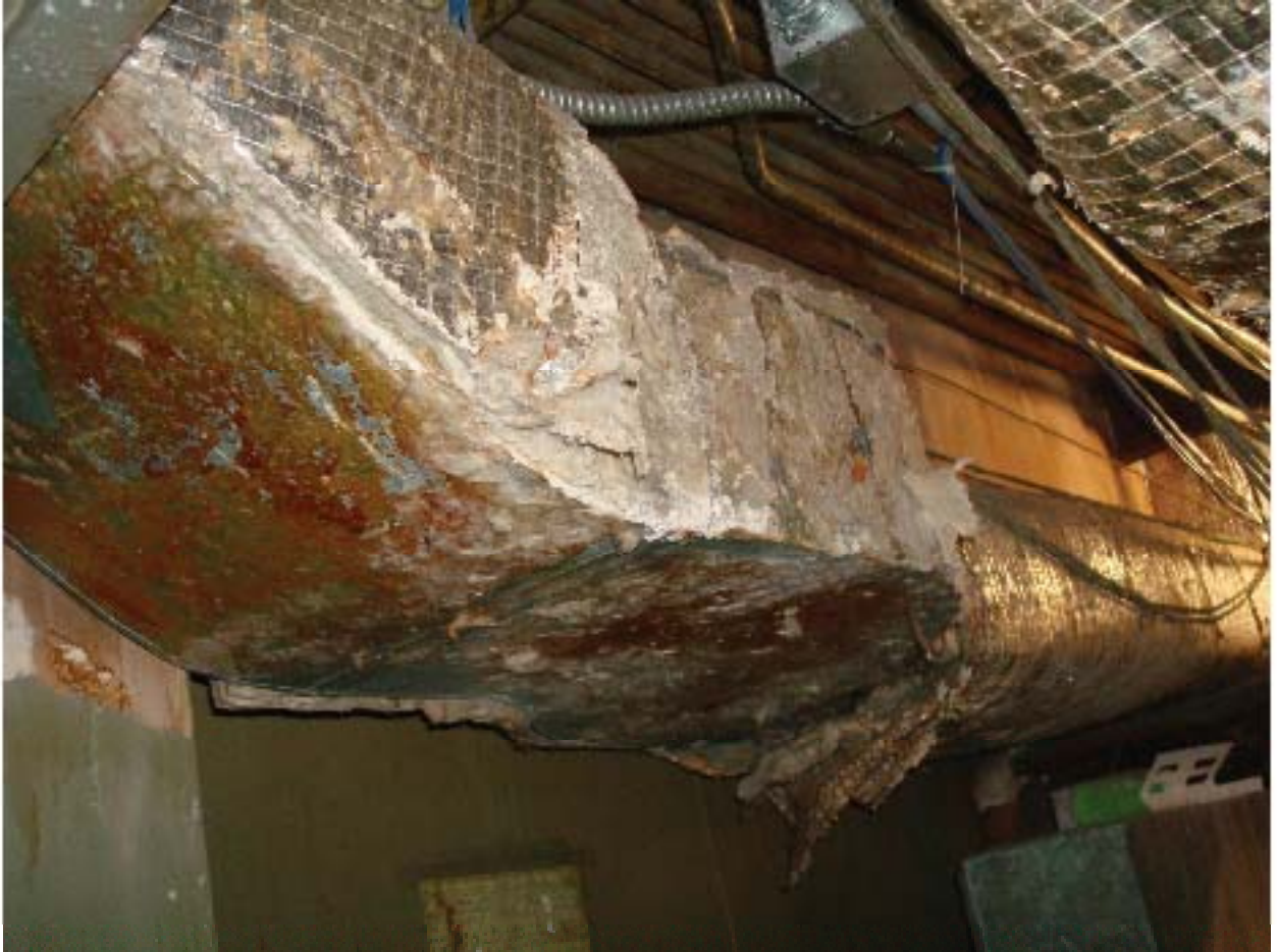
Rusting, decaying air ducts.
