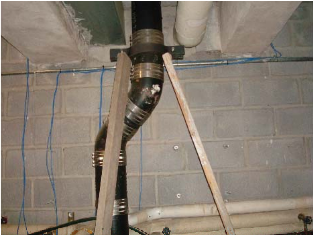
Repairs to these pipes were held together by pieces of wood.
