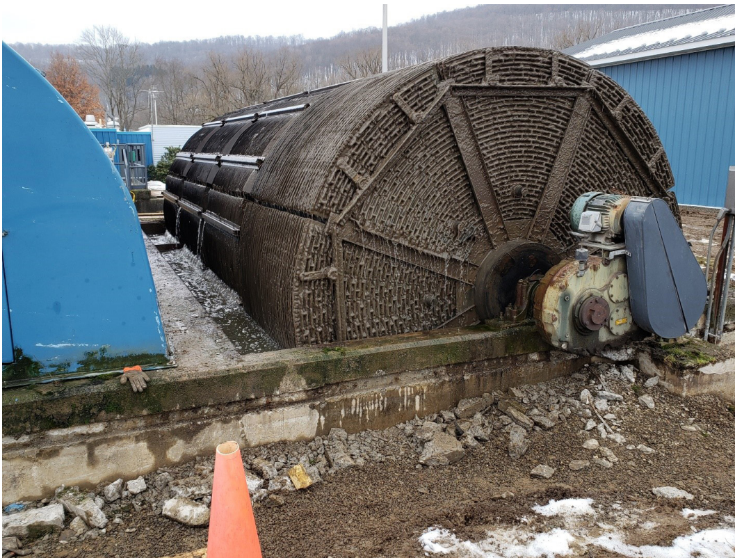
Figure 1: RBC in Need of Repair
