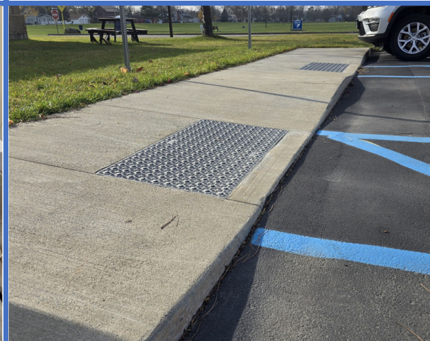
There are no level landings at the top of the curb ramps on the accessible route from the Library parking lot.
