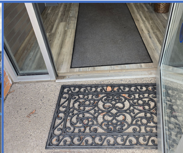
Mats at the Highway Department entrance should be secured or removed to minimize tripping hazards.
