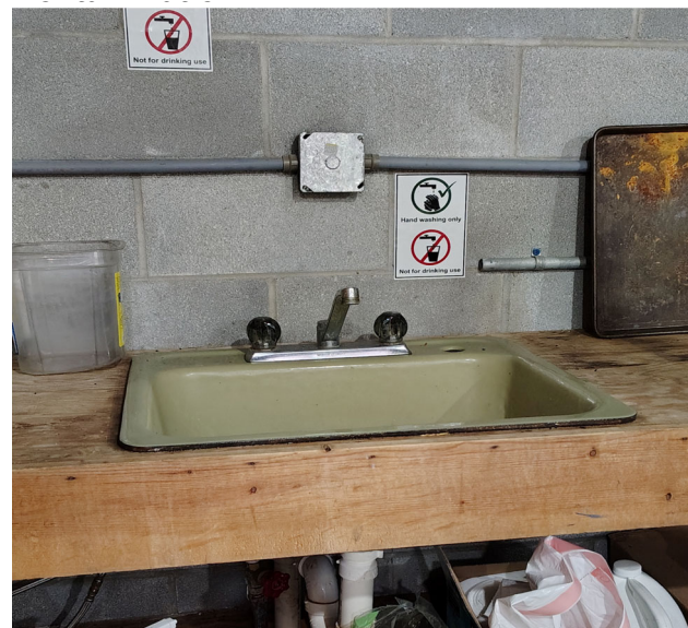
FIGURE 2: Concession Stand Sink Not Sampled and Tested For Lead Contamination a
