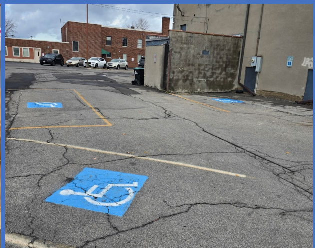
No van accessible parking and accessible aisles are not marked at the VFW Hall.
