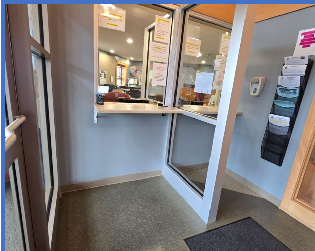
Service counter without an accessible portion no higher than 36 inches at Recreation.
