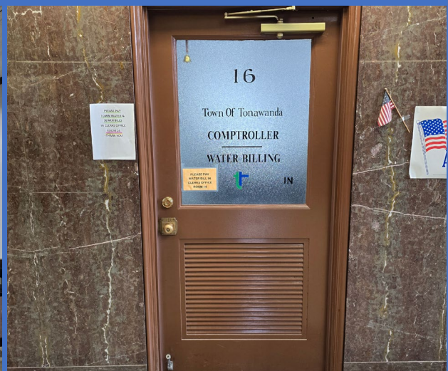
Signs at interior office (Town Comptroller's office pictured) without raised lettering and Braille mounted on the latch side of the door.
