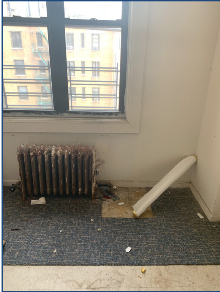
Regents heating risers: damage from flooding
