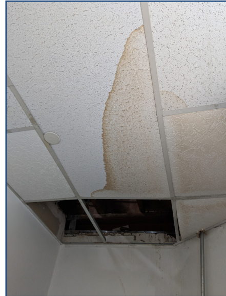
Park Slope roof replacement: water leaks in the art studio
