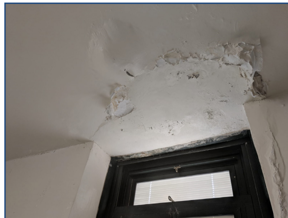
Jamaica exterior renovation: this room is off-limits due to water leak damage
