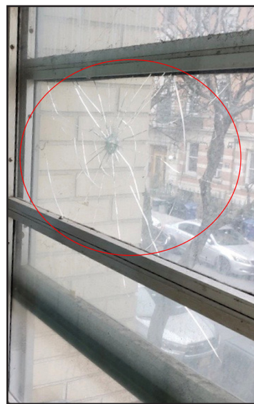
Image 5: Cracked window pane
