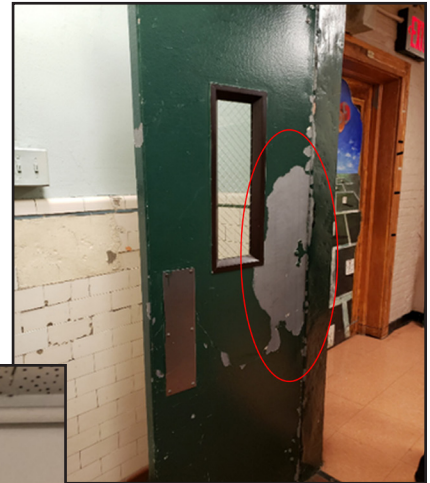
Image 2: Peeling paint on Brooklyn classroom door
