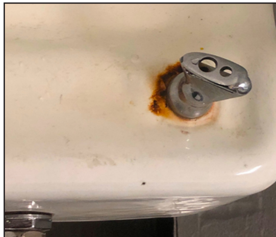
Image 18: Rust on base of water spout
