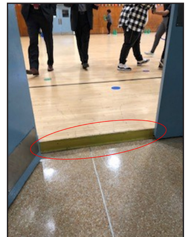
Image 16: Uneven gymnasium floor
