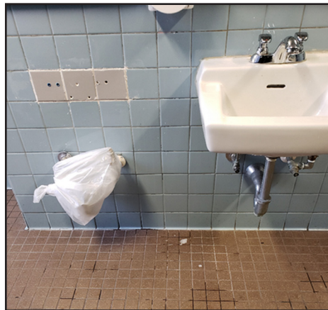
Image 15: Missing wash basin
