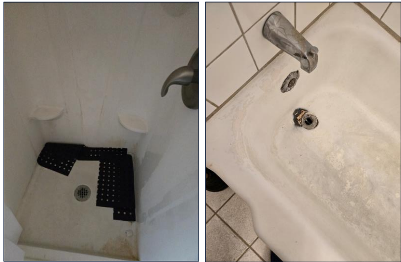
Mold in bathrooms.
