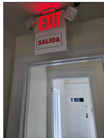
Spanish exit sign not illuminated at a CBRP provider.
