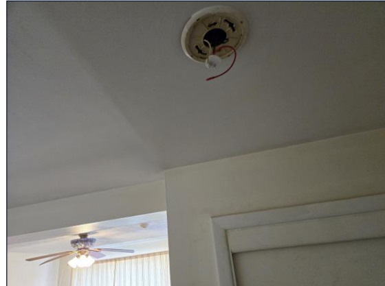
Disabled smoke detector observed at a CBRP provider.
