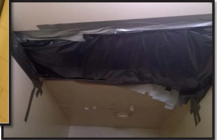
Trash bag and duct tape ceiling repair (Jennie A. Clarke family shelter, Manhattan)
