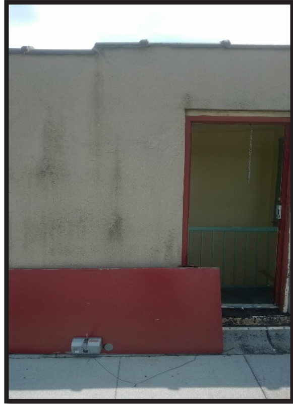
Detached door allowing unsecured roof access (Community Housing Innovations family shelter, Westchester County)
