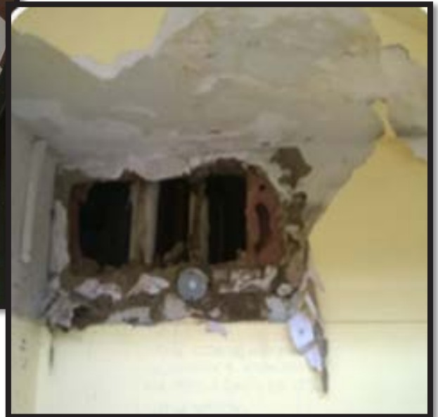
Wall with water damage and unrepaired hole (Kingsboro Psychiatric Center, Building 8 men's shelter, Brooklyn)
