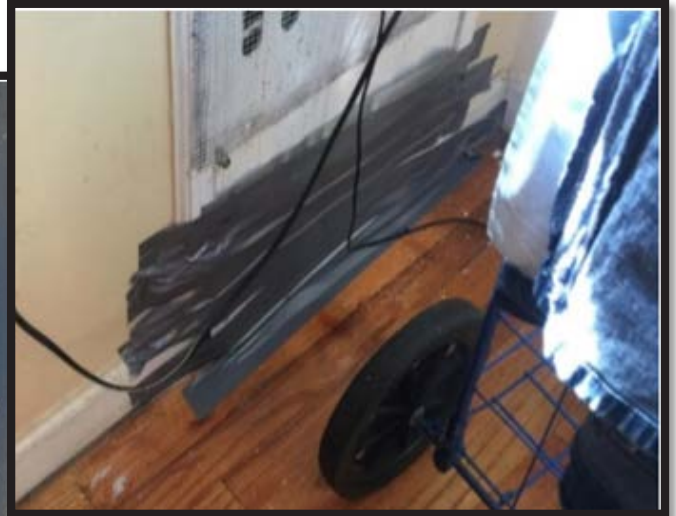
Vents taped over to prevent vermin access (Kingston Family Residence, Brooklyn)
