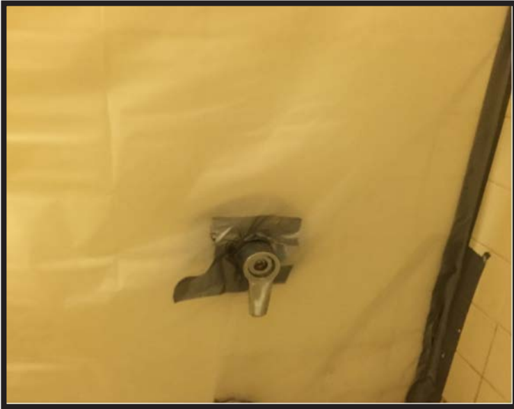
Shower fixture/wall repaired with heavy-duty plastic sheeting and duct tape (St. John's Place family shelter, Brooklyn)
