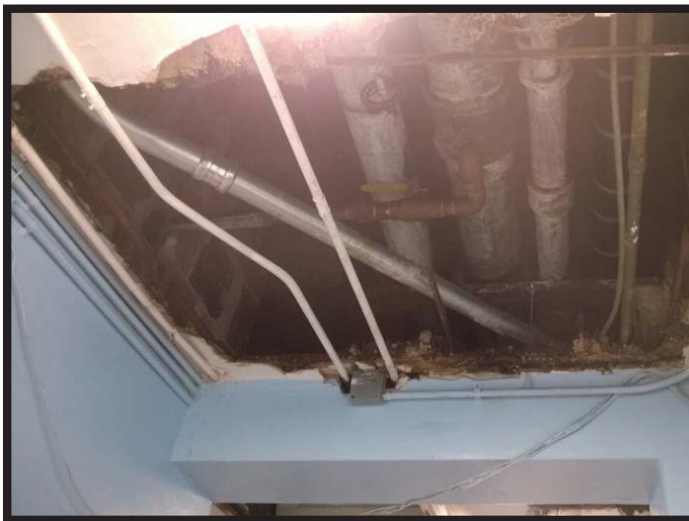
Missing ceiling (Bellevue 30th Street Men's Shelter, Manhattan)
