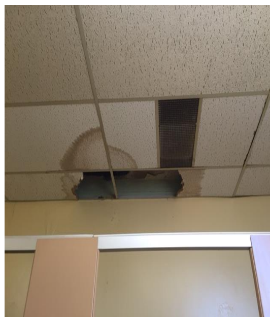
WATER DAMAGED CEILING TILES
