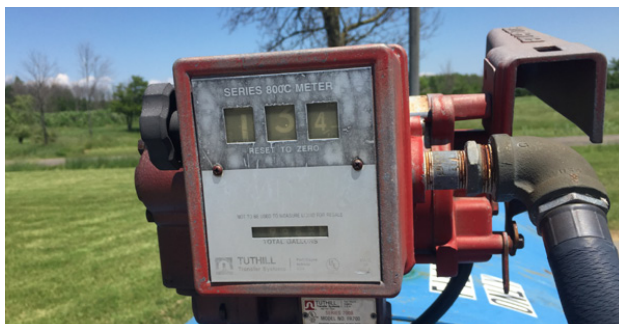
Photos: 2,000 gallon reserve fuel tank at Hamburg Highway Department
